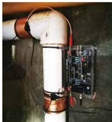
Vulcan S10安装在总出水管道上
